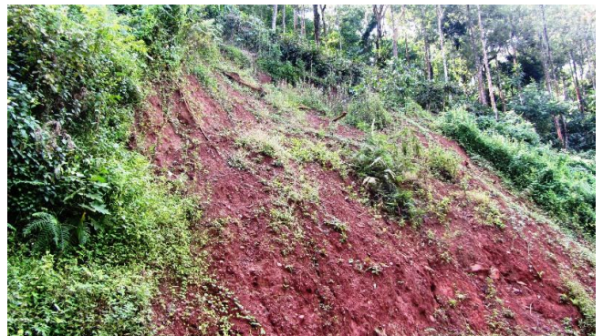
Photo: 4 Slope failure (Chittalli-Madikere road)
