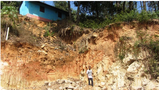
Photo: 3 Precariously placed house due to Extensive road cut (Virajpet hill)
