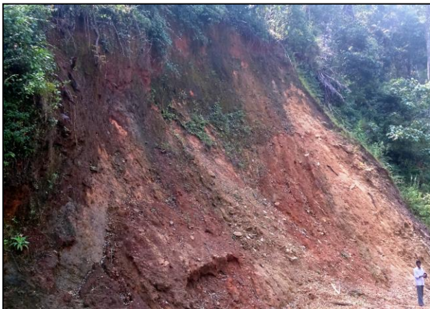
Photo:3 Debris slide on Hacchinadu – Galibidu road, T.S. No. 48P/11.
