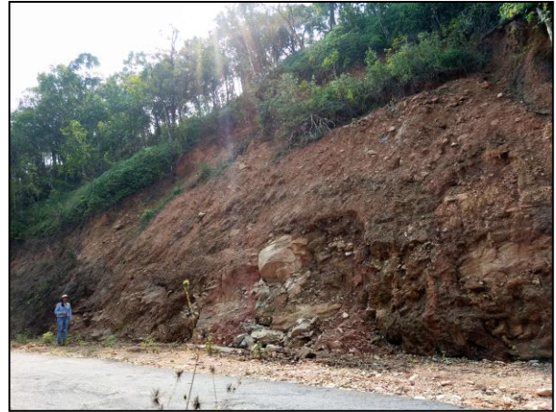
Photo:2 Debris slide on Hacchinadu – Galibidu road, T.S. No. 48P/11.
