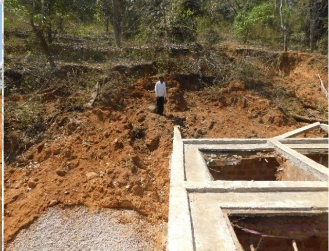
Photo 3. 2f Debris slide near Barahmeswara village (Lat: 13°57'15.49"Long: 75°04'44.32")
