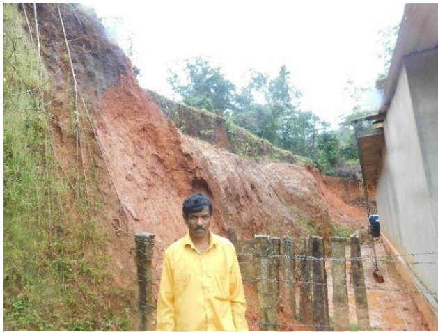
Photo 4.1a Settlement on modified slope (Lat: 13°47' 3.1" Long: 75° 20' 54.6")
