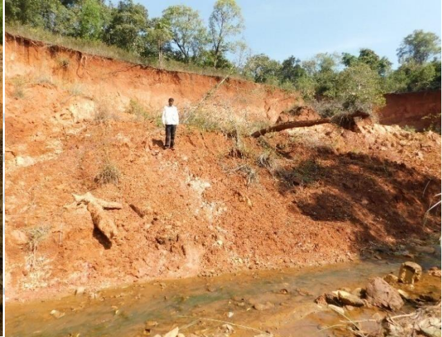
Photo 3. 2d Debris slide near Kannuru village (Lat: 13°55'6.1"Long: 75°11'01")
