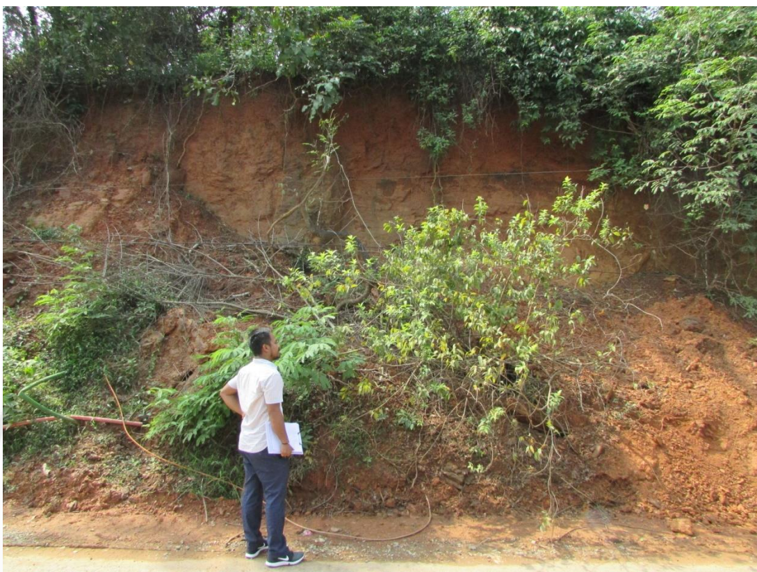
Fig. 3.3: Active debris slide along Sanverdam - Siroda road (slide Name: GOA/SG/48I03/2019/03).
