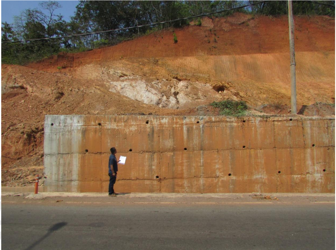
Fig. 4.4: Extensive Slope Cut along Ponda – Molen road near Ponda. The height of the retaining structures should be increased.
