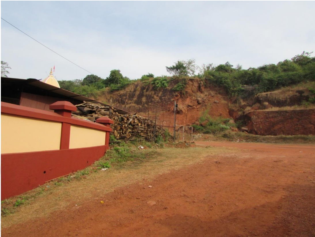
Fig. 4.6: Extensive Slope Cut just behind the Sai Baba Temple at Borim. Retaining structures should be provided to the unsupported slopes.
