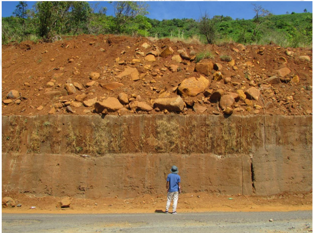
Fig. 3.6: Reactivated debris slide along Chorla Ghat road (slide Name: GOA/NG/48I02/2019/18).
