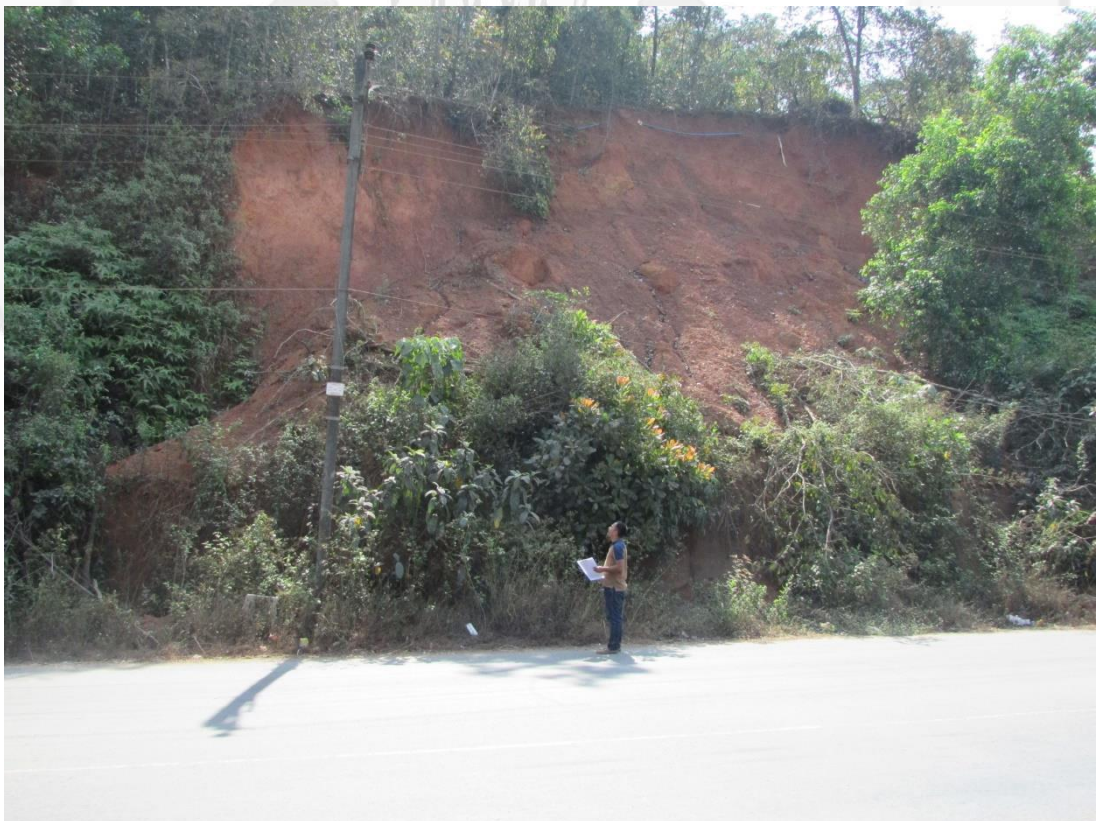
Fig. 3.8: Reactivated debris slide along Borim - Ponda bypass road (slide Name: GOA/SG/48I03/2020/23).
