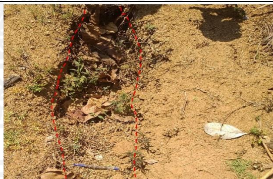
Fig. 6.3b Transverse crack at downslope of the Ambatty road
