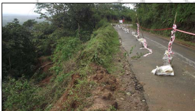
Photo 23: View of landslide near Kattalekadu on SH-89 between Madikeri-Chettali.
