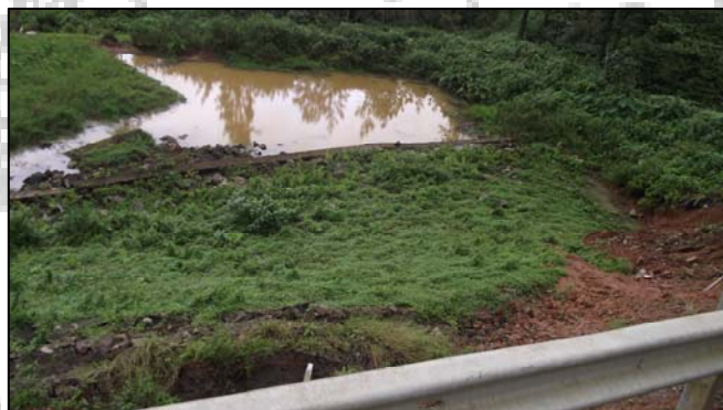
Photo 22: Movement of toe wall after subsidence on SH-88 near Sinchona estate (Boyikere) between Madikeri – Suintikoppa.
