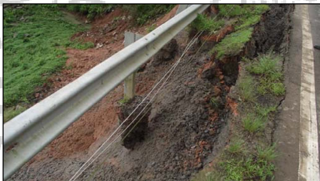
Photo 21: Subsidence on SH-88 near Sinchona estate (Boyikere) between Madikeri – Suintikoppa.
