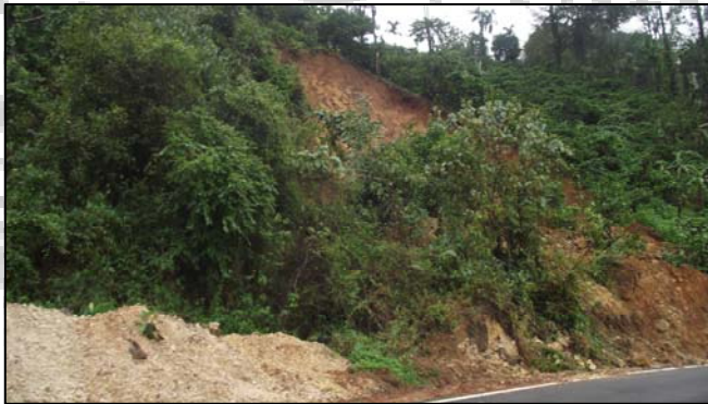
Photo 10: View of slide Landslide on SH-88 between Madikeri-Samapje
