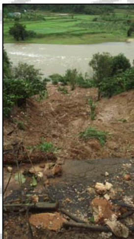
Photo 13: Runout of Landslide on Makandur-Mukkodlu tantipal road in to Kalur Nala.
