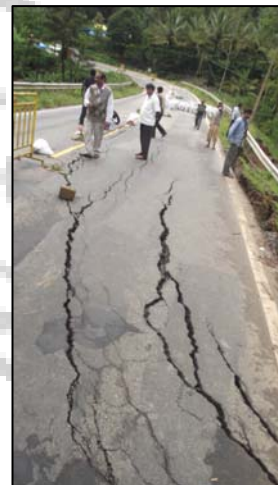
Photo 20: Cracks on SH-88 near Sinchona estate (Boyikere) between Madikeri – Suintikoppa.
