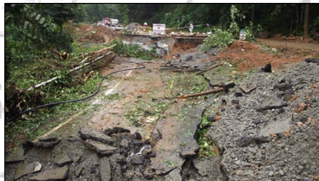
Photo 30: View of subsidence on SH-88 near Koynad between Madikeri -Sampaje.
