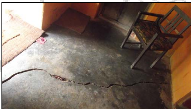
Photo 5: Cracks seen in house of Smt. Janaki in Makandur village.
