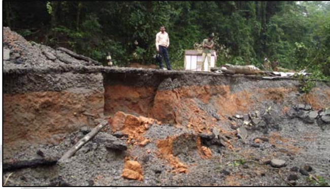
Photo 31: View of subsidence on SH-88 near Koynad between Madikeri –Sampaje.
