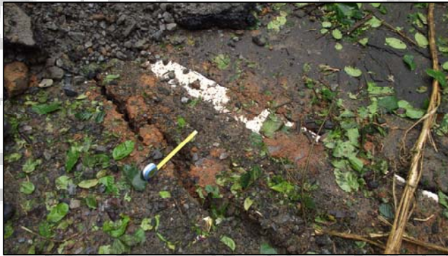
Photo 33: Ground cracks on SH-88 Near Koynad.
