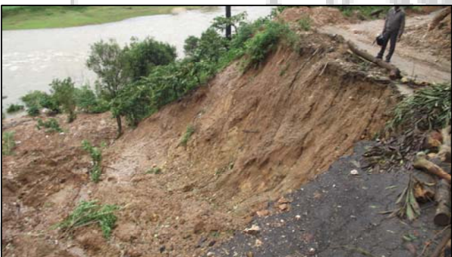
Photo 11: View of Landslide on Makandur-Mukkodlu tantipal road.
