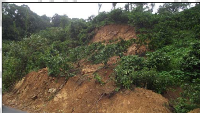
Photo 9: View of Landslide on SH-88 between Madikeri-Samapje
