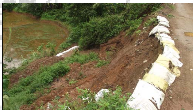
Photo 18: View of landslide near Makandur village, Sinchona estate road.
