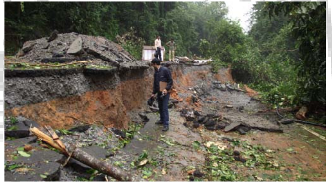
Photo 34: View of subsidence on SH-88 near Koynad between Madikeri –Sampaje.
