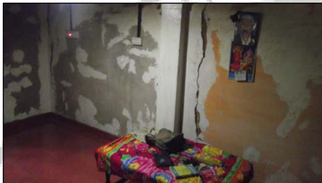
Photo 7: Cracks seen in house of Smt. Janaki in Makandur village.
