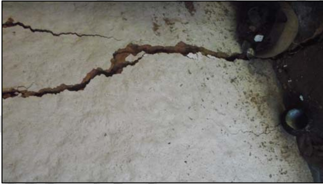
Photo 1: Cracks seen in house of Shri. Jayaprakash in Mannangeri village.
