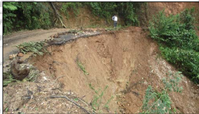
Photo 12: View of Landslide on Makandur-Mukkodlu tantipal road.
