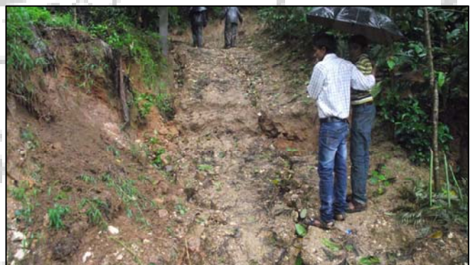
Photo 6: Subsidence observed Upstream of Smt. Janaki house.
