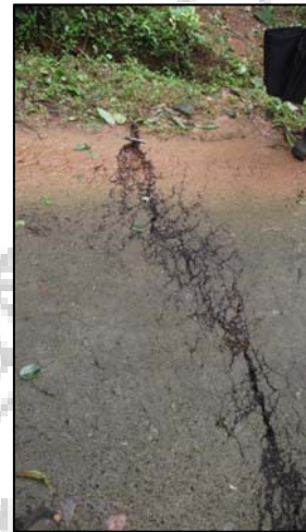
Photo 4: Cracks seen road leading to School in Mannangeri village.
