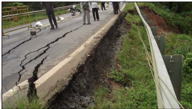
Photo 19: Cracks on SH-88 near Sinchona estate (Boyikere) between Madikeri – Suintikoppa with subsidence.
