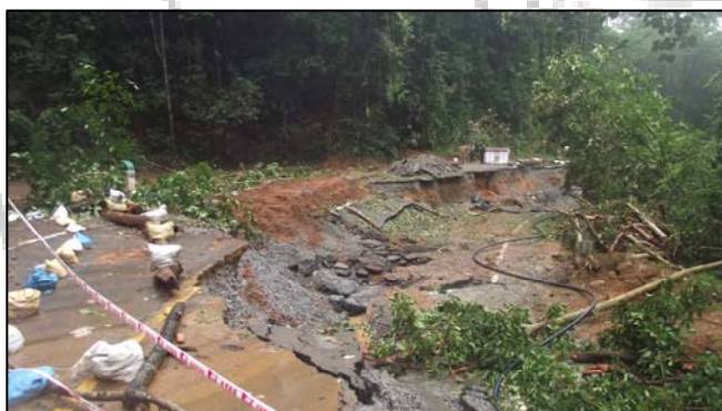
Photo 29: View of subsidence on SH-88 near Koynad between Madikeri -Sampaje.
